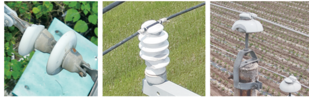
图2 破损 Fig.2 Damage
